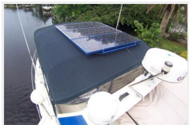
450 Watt Solar Panel Array
