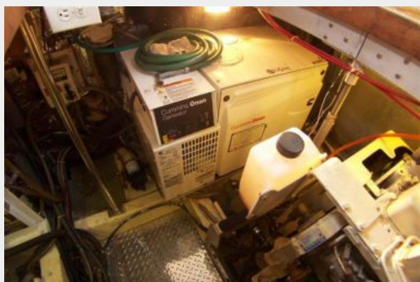
ONAN Genset with sound enclosure
