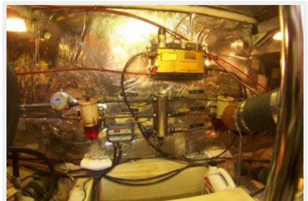
Engine Room - aft
