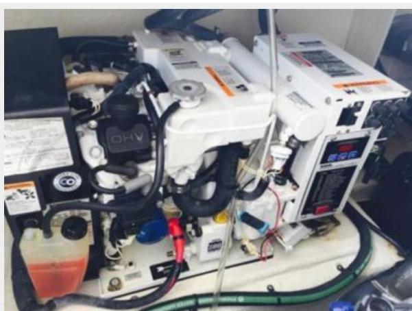
5KW Kohler Generator
