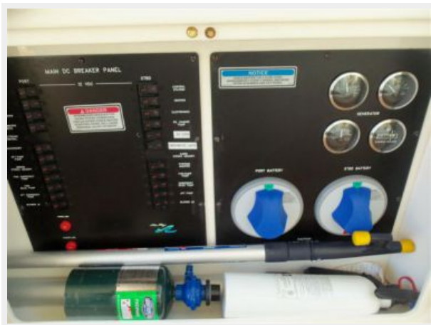
Cockpit Electrical Panel
