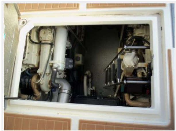
Engine Room Access
