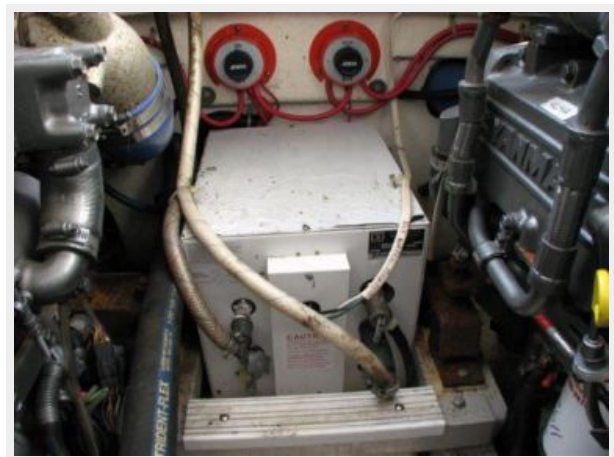
Engine & Mechanical Equipment 4 - Engine Room
