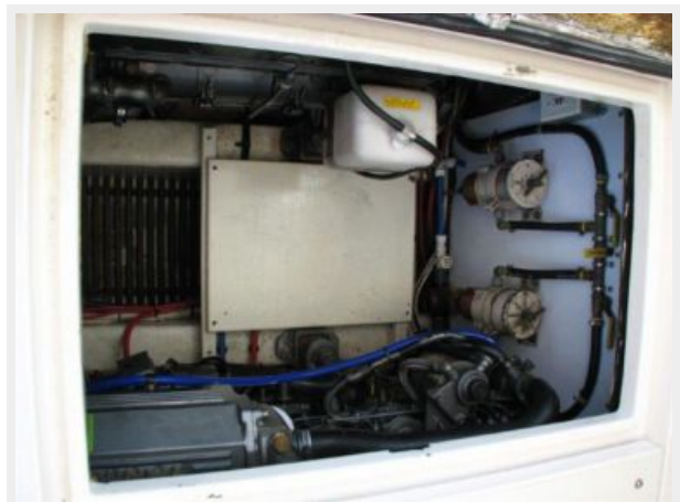
Engine & Mechanical Equipment 3 - Engine Room
