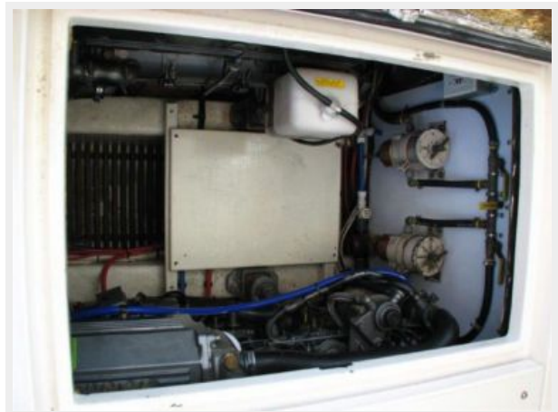
Engine & Mechanical Equipment 3 - Engine Room
