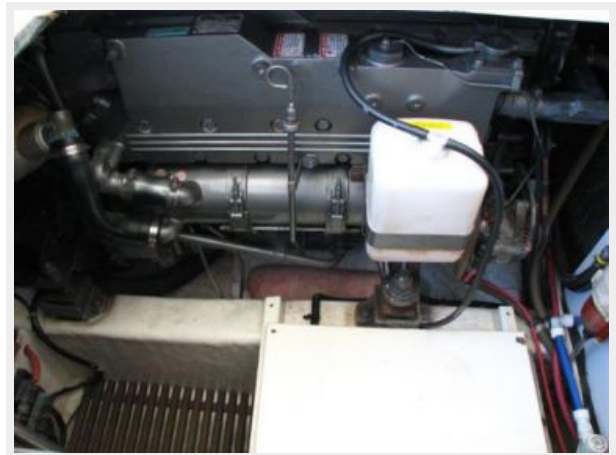
Engine & Mechanical Equipment 1 - Port Engine
