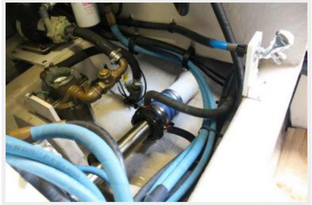
Starboard Shaft Seal, AC Intake & Fresh Water Supply
