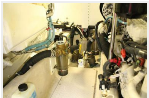
Clean Bilges & Raw Water Strainers
