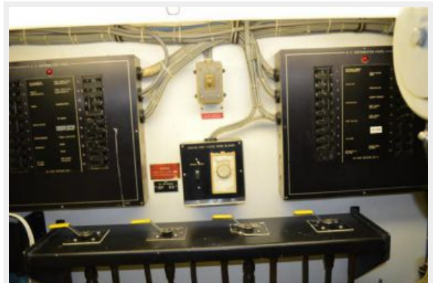
Breakers & Fuel Manifold
