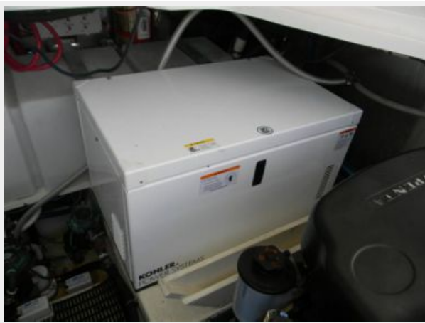
Generator with Soundshield
