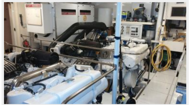
Engine Room from Stbd Side
