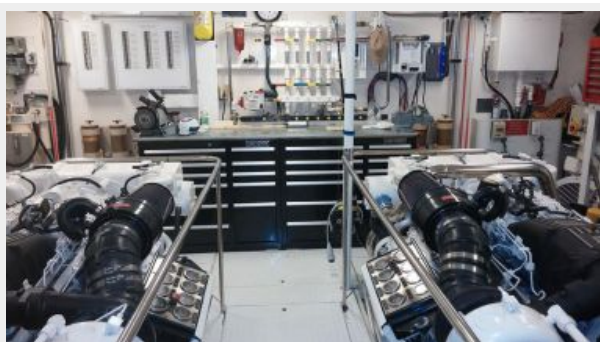
Engine Room Looking FWD
