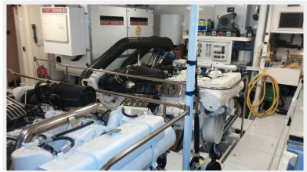
Engine Room from Stbd Side
