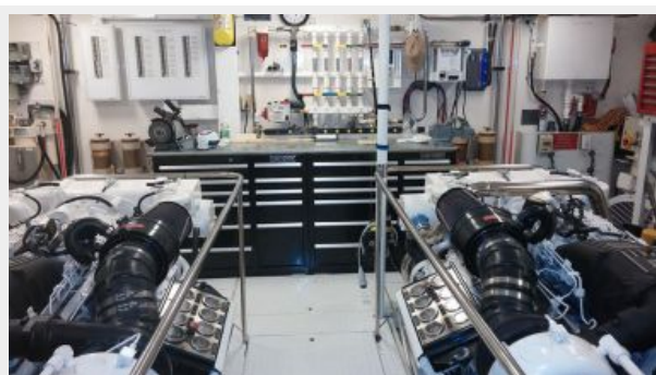
Engine Room Looking FWD
