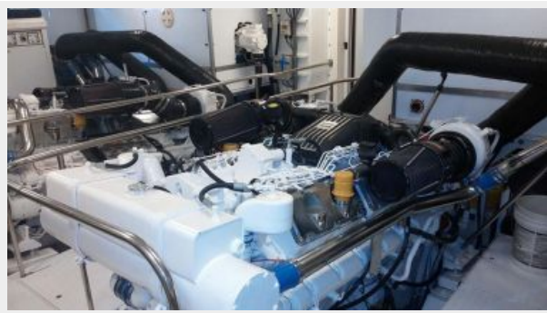
Engine Room Port Side
