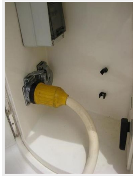
Shore Power Connection
