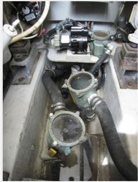
Engine Room - forward
