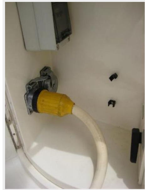
Shore Power Connection
