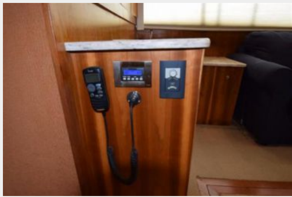
Salon VHF/ AC controls
