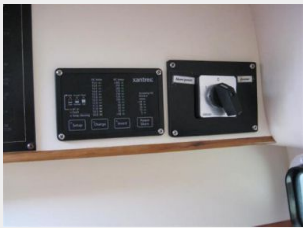
Xantrex Inverter, 30 amp Shore Power Connection
