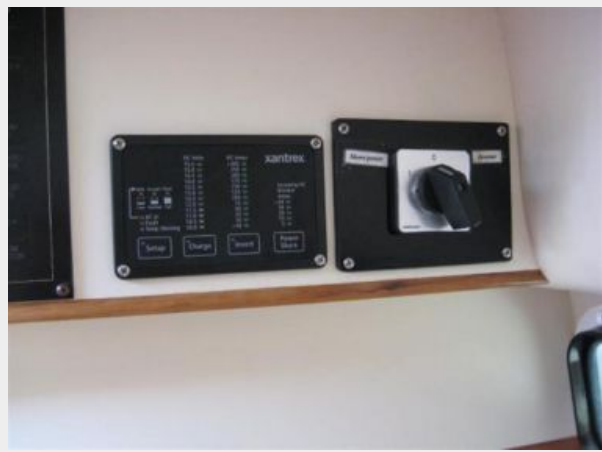
Xantrex Inverter, 30 amp Shore Power Connection
