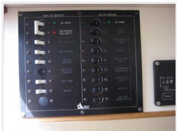
Electrical Breaker Panel
