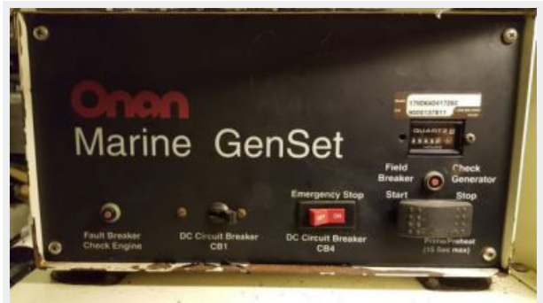
3945 Hours on Genset
