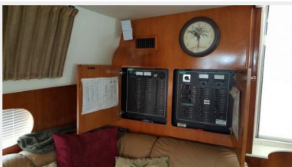
Main Distribution Panel
