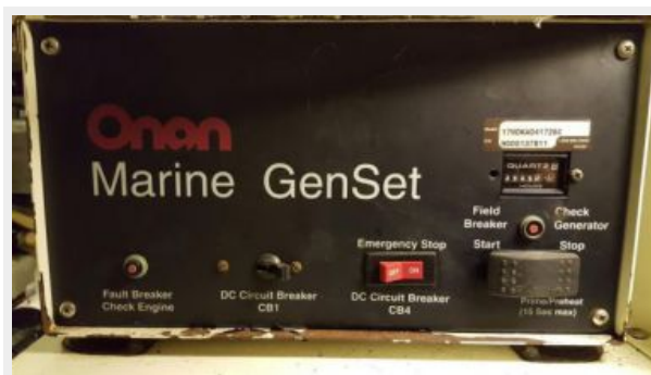
3945 Hours on Genset
