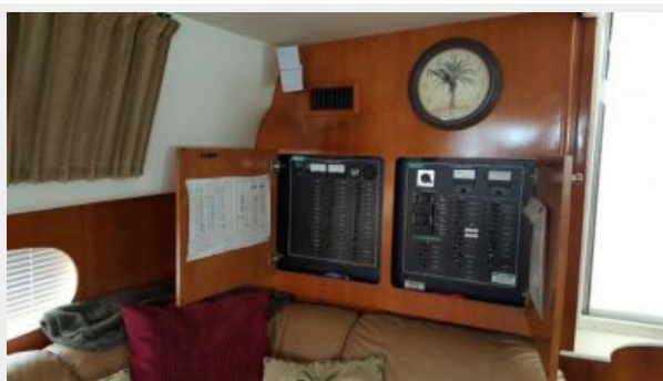
Main Distribution Panel
