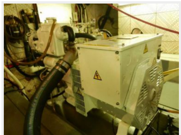
8.5 kw Phasor generator
