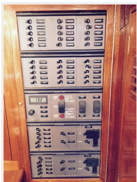
Front of Electrical Panel
