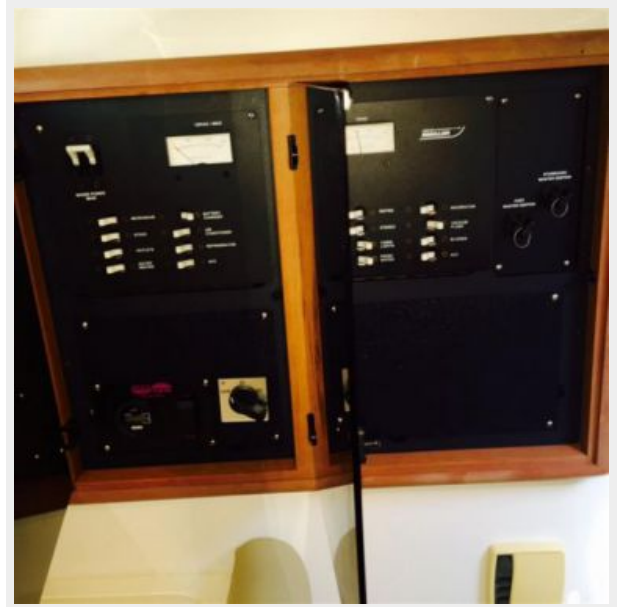
Main Distribution Panel
