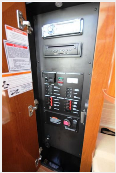
Main Distribution Panel
