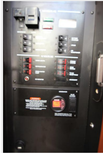
38 Hours on Genset
