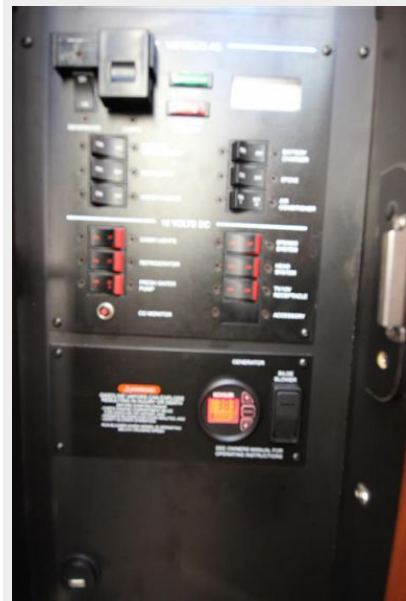
38 Hours on Genset
