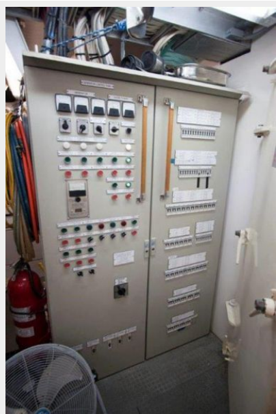
Machine Room Electric
