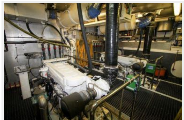
Engine Room Forward
