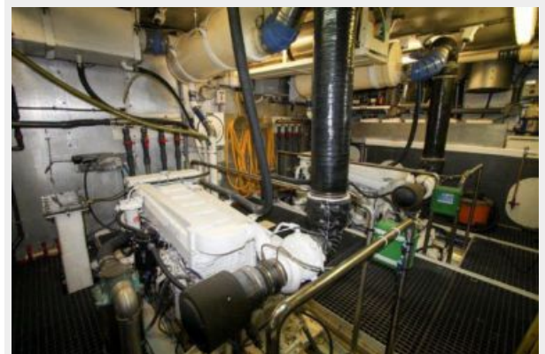
Engine Room Forward
