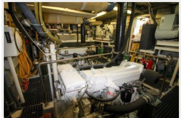
Engine Room Aft
