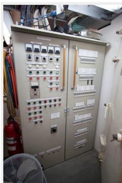
Machine Room Electric
