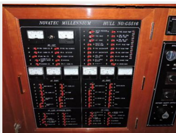
Shore Power Panel
