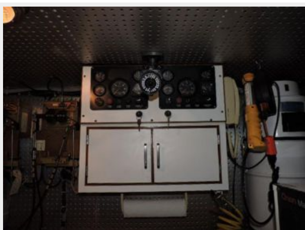
Engine Room Controls
