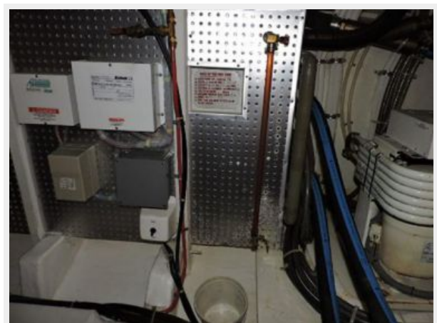
Fuel Tank and Site Gauge
