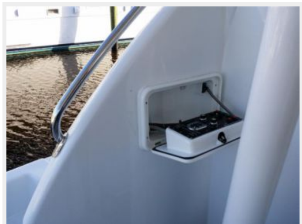
Aft Control Station
