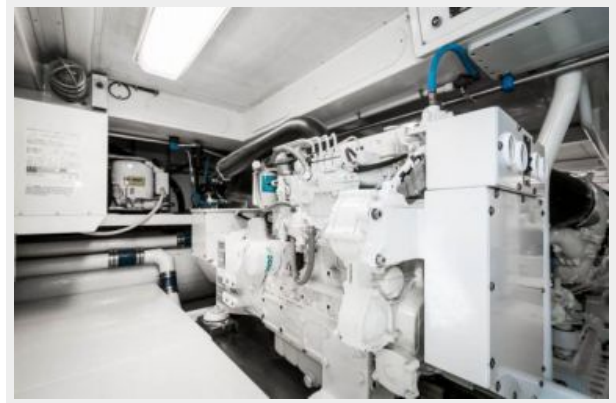
Badonkadonk Merritt 2000 Engine Room Port Generator
