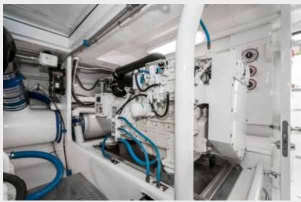
Badonkadonk Merritt 2000 Engine Room Starboard Generator
