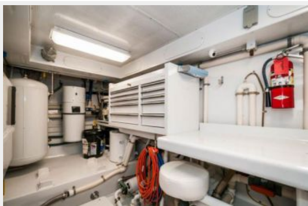
Badonkadonk Merritt 2000 Engine Room Work Bench
