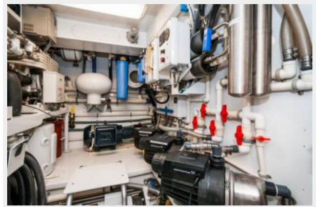
Badonkadonk Merritt 2000 Engine Room Water Maker
