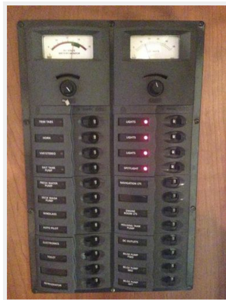
Electrical Panel Detail
