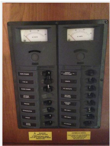
Electrical Panel Detail
