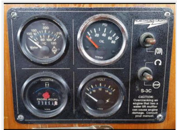
49' Marine Trader Generator Panel
