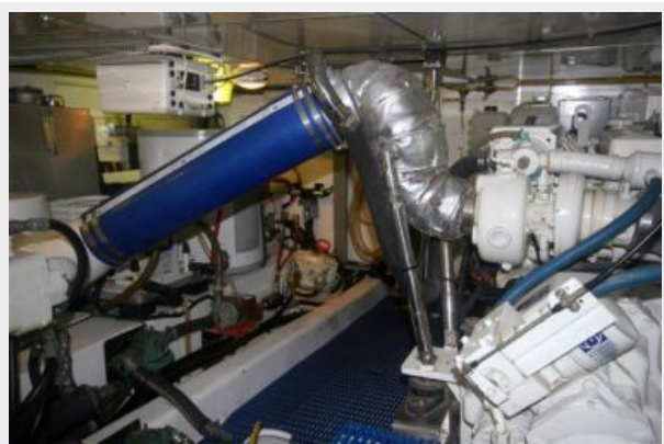
Engine Room Port
