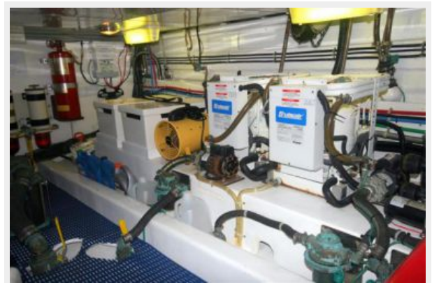
Engine Room Starboard
