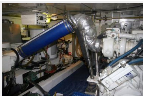
Engine Room Port
