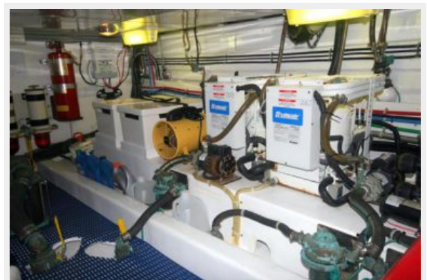
Engine Room Starboard
