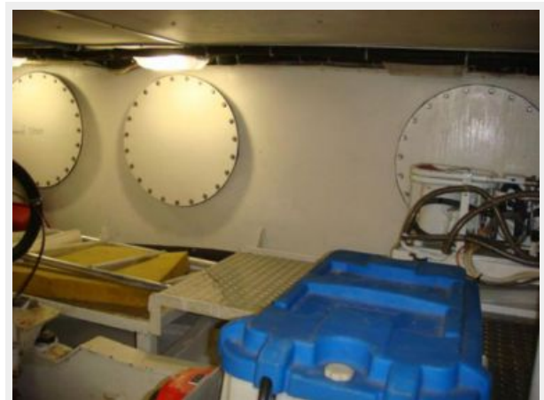
39' Neville Trawler engine room starboard
