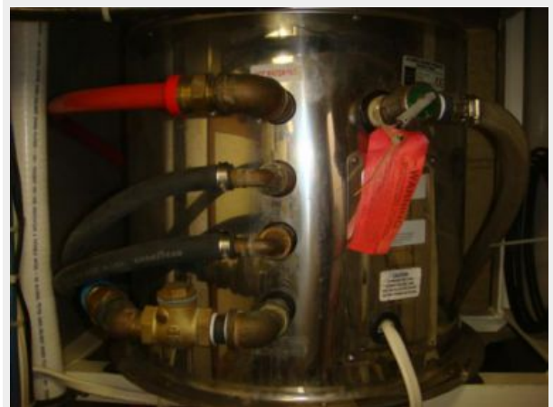
39' Neville Trawler water heater
