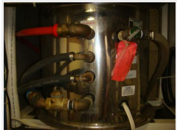
39' Neville Trawler water heater
