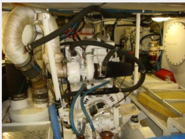
39' Neville Trawler engine room forward
