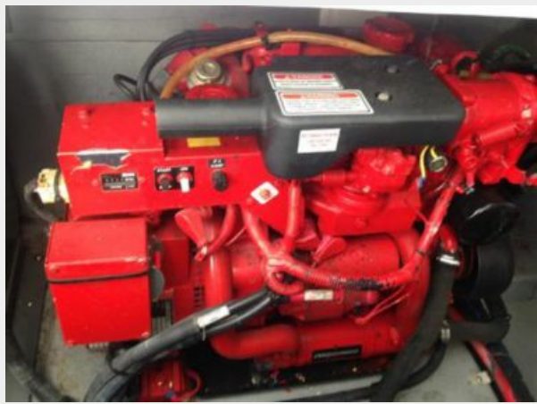
5.0 kW Westerbeke Generator
