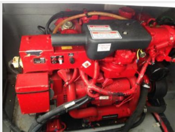
5.0 kW Westerbeke Generator
