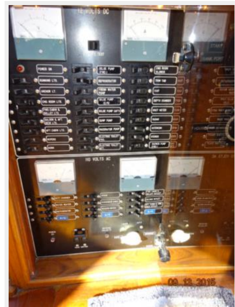
43' Marine Trader electrical panel
