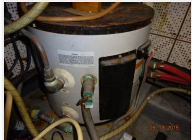
43' Marine Trader water heater
