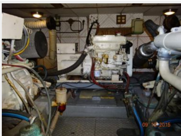
43' Marine Trader engine room aft
