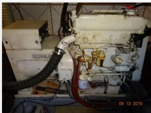
43' Marine Trader generator
