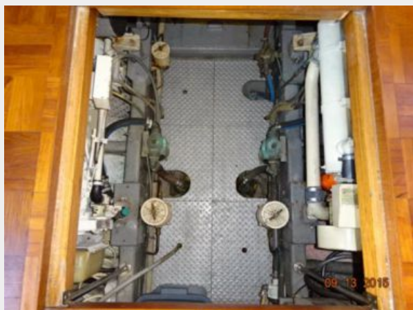
43' Marine Trader engine room access
