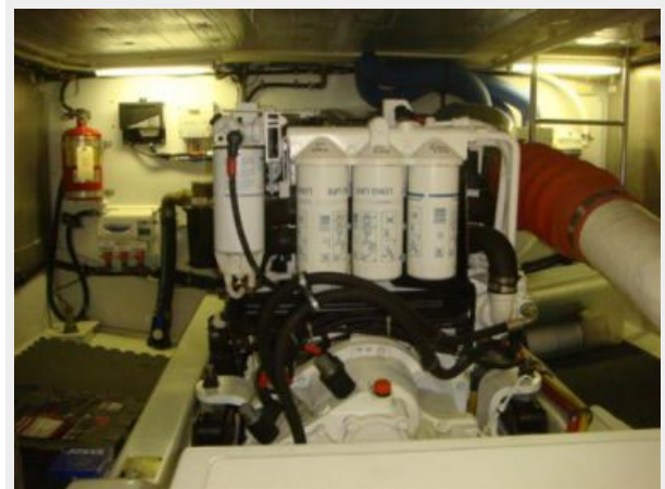
41' American Tug engine room forward
