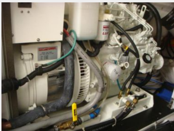
41' American Tug generator
