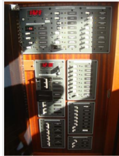
41' American Tug electrical panel
