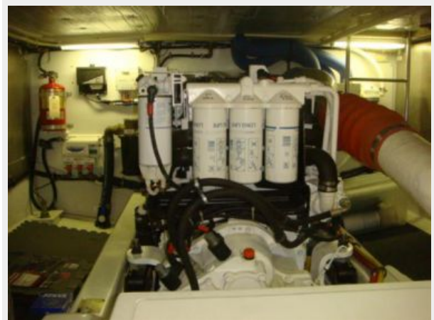
41' American Tug engine room forward
