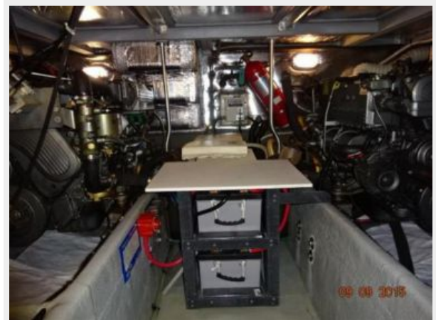
43' Mainship engine room aft
