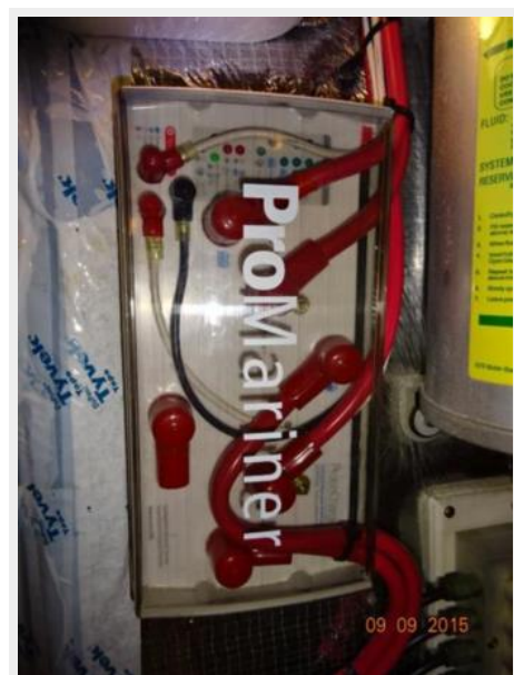
43' Mainship battery isolator
