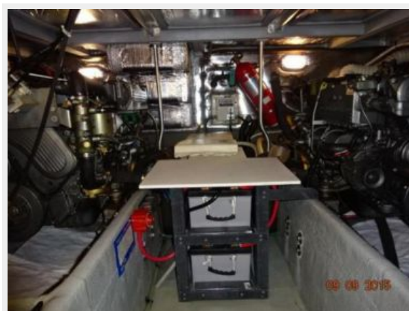
43' Mainship engine room aft
