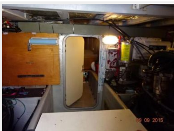
43' Mainship engine room forward
