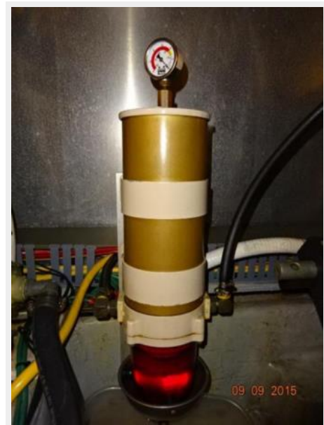
43' Mainship starboard Racor fuel filter
