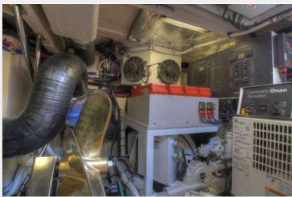
Engine Room w/ Spare Props
