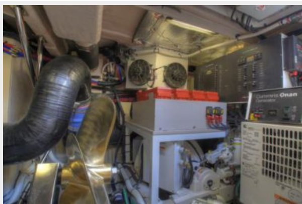
Engine Room w/ Spare Props
