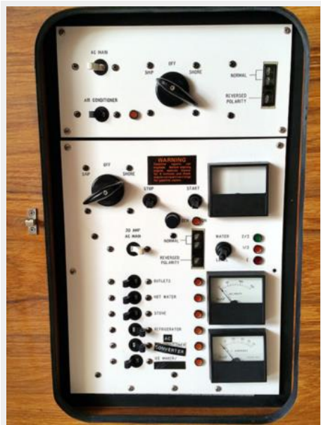
34' Sea Ray Electrical Panel
