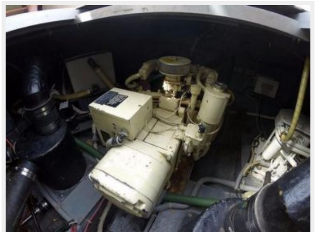
34' Sea Ray Generator
