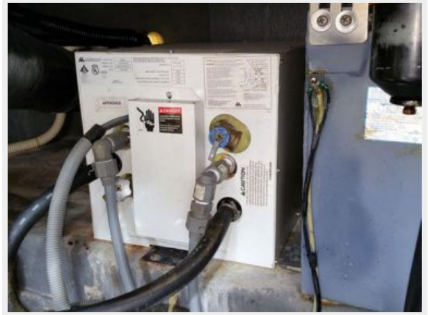
34' Sea Ray Water Heater
