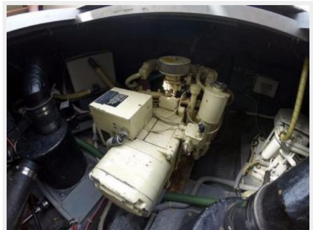
34' Sea Ray Generator
