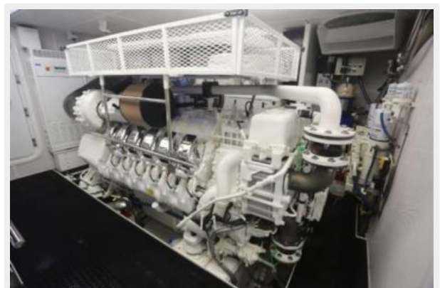
Port Engine with Custom Storage Rack Above
