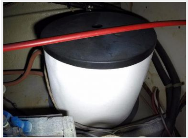
36' Chris Craft Water Heater
