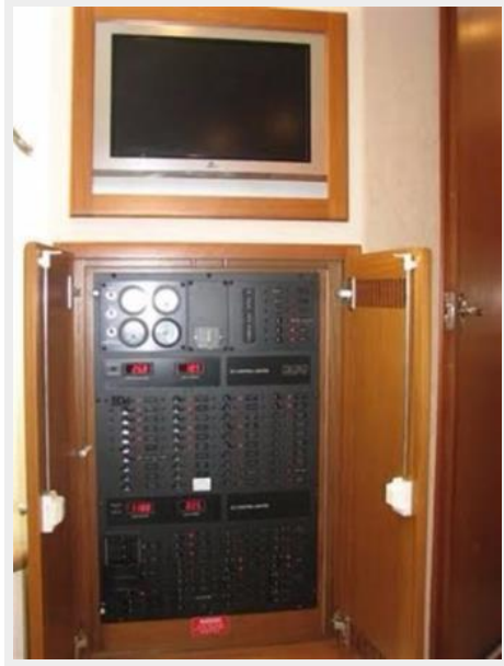
Salon TV & Breaker Panel
